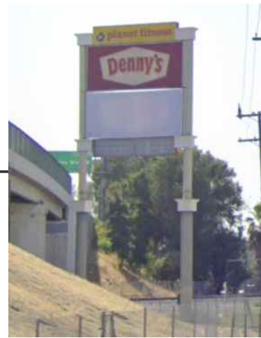
Existing pylon at 28'-0" w X ± 67'-0" ht Shall be fully removed prior to Replacement Pylon installation.
